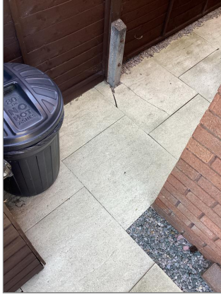
Photo - 16 Cracked and uneven paving
