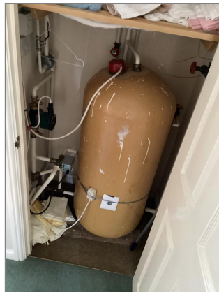
Photo - 15 Hot water cylinder
