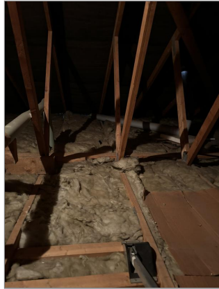
Photo - 5 Insulation minimal
