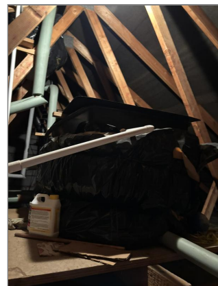
Photo - 13 Water tank
