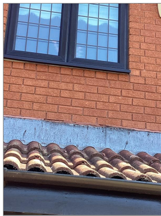
Photo - 1 Mortar pointing missing to flashing
