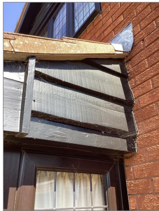
Photo - 4 Slightly weathered joinery
