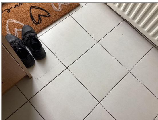
Photo - 10 Cracking to tiles
