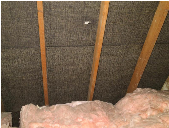
Photo - 9 Damage to sarking felt
