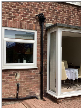
Photo - 15 Rear waste pipe
