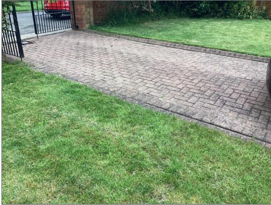
Photo - 18 Uneven driveway
