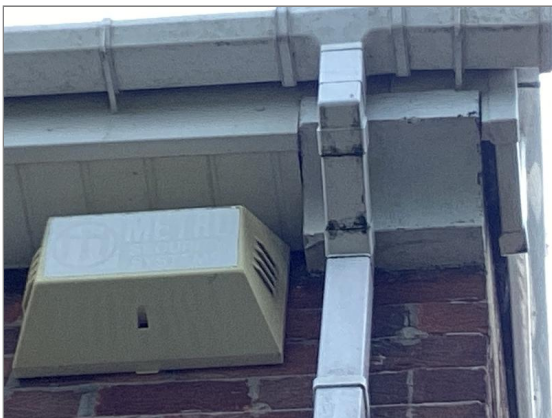
Photo - 6 Staining to joints
